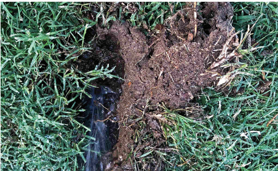
SDI tubing can be damaged by aeration and cultivation equipment, which may limit the cultural practices available in areas irrigated by SDI. This section of dripline was punctured by an aerator. (Bernd Leinauer)
