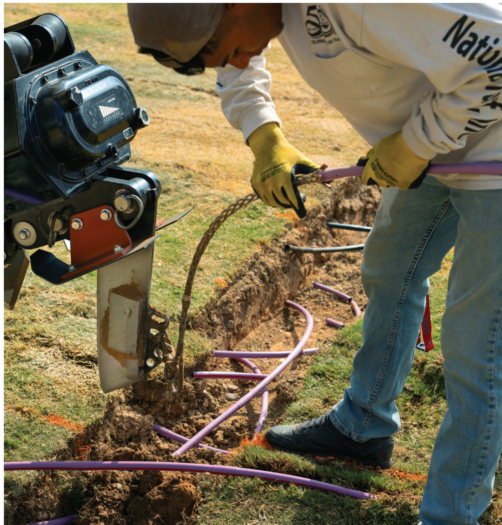
Installing SDI is more challenging and expensive over a given area of turf than installing overhead sprinklers. (USGA/Bill Hornstein)
