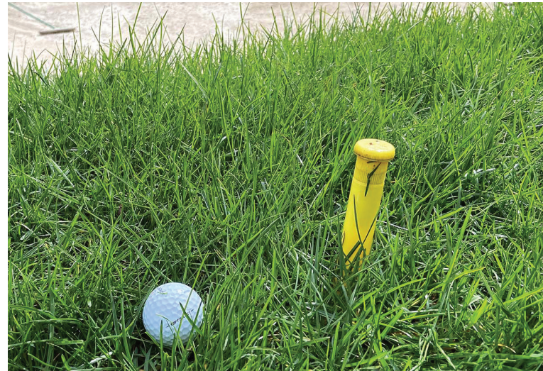
Installing a closed pop-up sprinkler at the end of a drip line allows you to see if the line is properly charged and coming on when expected.
